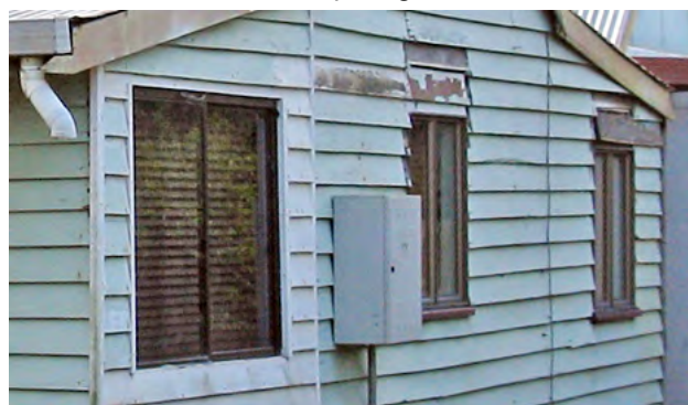
Side wall detail: Note the difference in weatherboard colour and trim location. The loose vertical cable where the roof indicates the rear verandah starts could from an underground telephone service. In other locations it might be connected to a lightning rod. The spaces above the middle and rear replacement windows have been roughly filled in with what looks like weatherboard. The front gutter (eavestrough) no longer has a vertical downpipe, perhaps removed when municipal authorities banned rainwater tanks.
