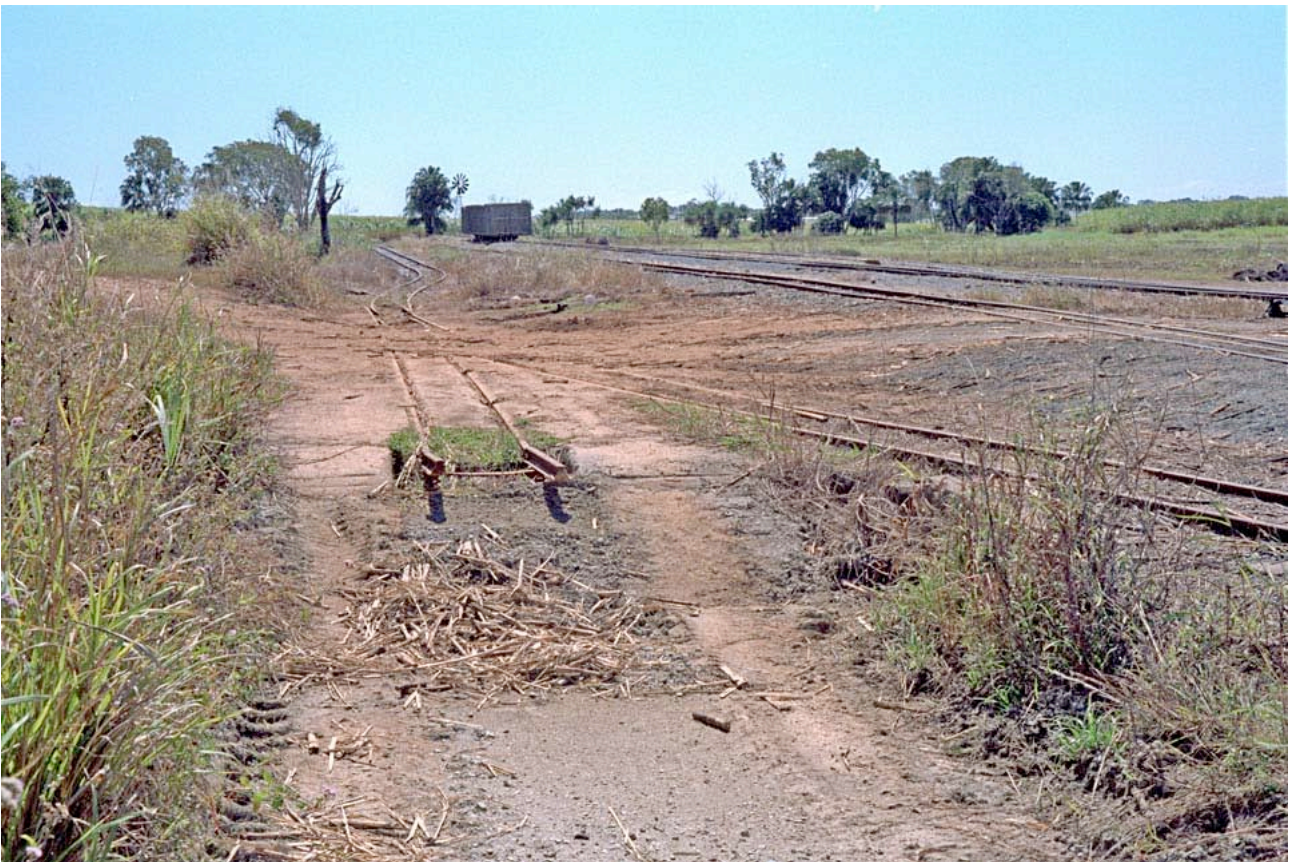
Tractor/truck dump on a line near Mackay clearly showing the different line elevations and grades. Lynn Zelmer, photographer.
