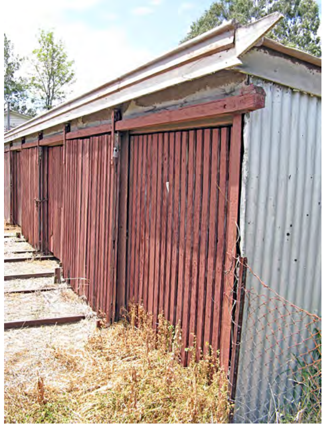
South end of the Mount Morgan fettler's shed, October 2008. Note the shape of the fascia board end and the painted sheathing. A door lock can be seen at the top of the first door, the lock on a door further along is at waist level..
