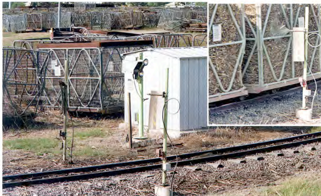
LEFT: Bin identification equipment at Mackay Sugar's Marian Mill, September 1990. Main picture left to right on posts are a washer unit for bin mounted barcodes, a barcode reader with lights, and a second washer.
