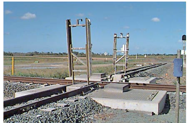
Drawbridge to allow cane railway to cross QR's mainline near Mackay. October 1997.
