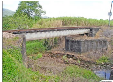
A narrow gauge does not imply lower standards, and modern bridges have to carry quite heavy loads for much faster moving trains than in the past.
