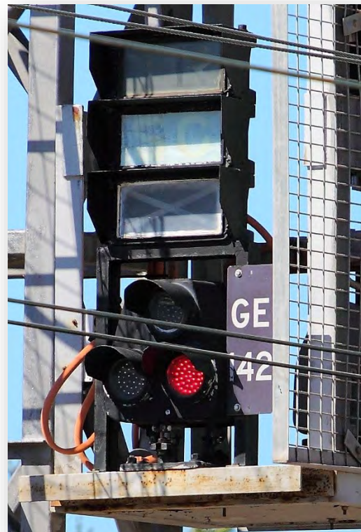
Position Light Signal with Route Indicators
