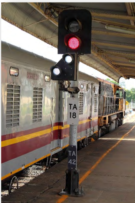
2 Aspect Sub Shunt Signal
