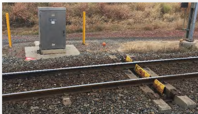
Dragging Equipment Detector (DED)
