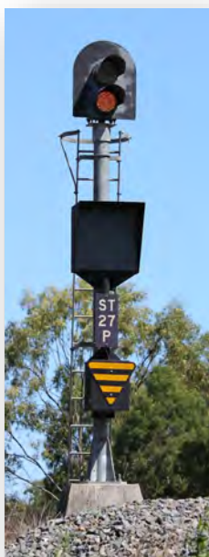
DSI fitted below an Approach Signal
