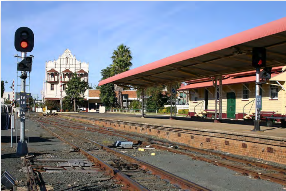
Mainline and Loop Starting Signals
