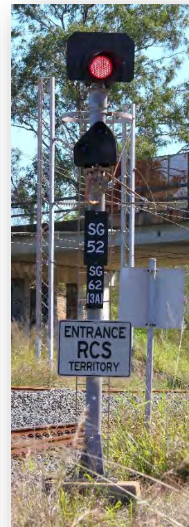
Single Aspect Red with Sub Shunt Signal
