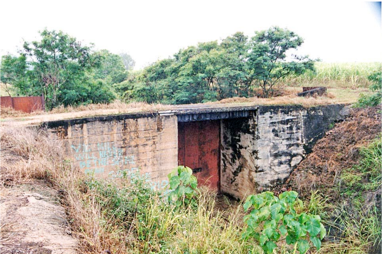
The floodgate installed at Herbert River crossing on Victoria Mill's system.
